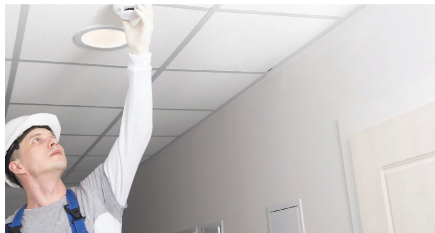
Firebrand technician inspecting a fire detector
