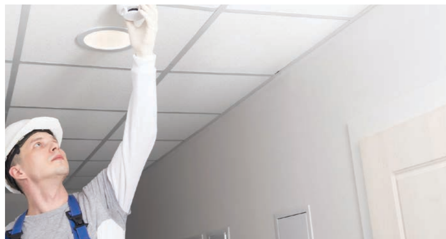
Firebrand technician inspecting a fire detector
