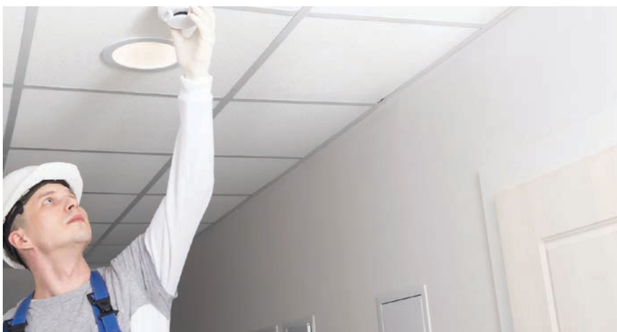
Firebrand technician inspecting a fire detector
