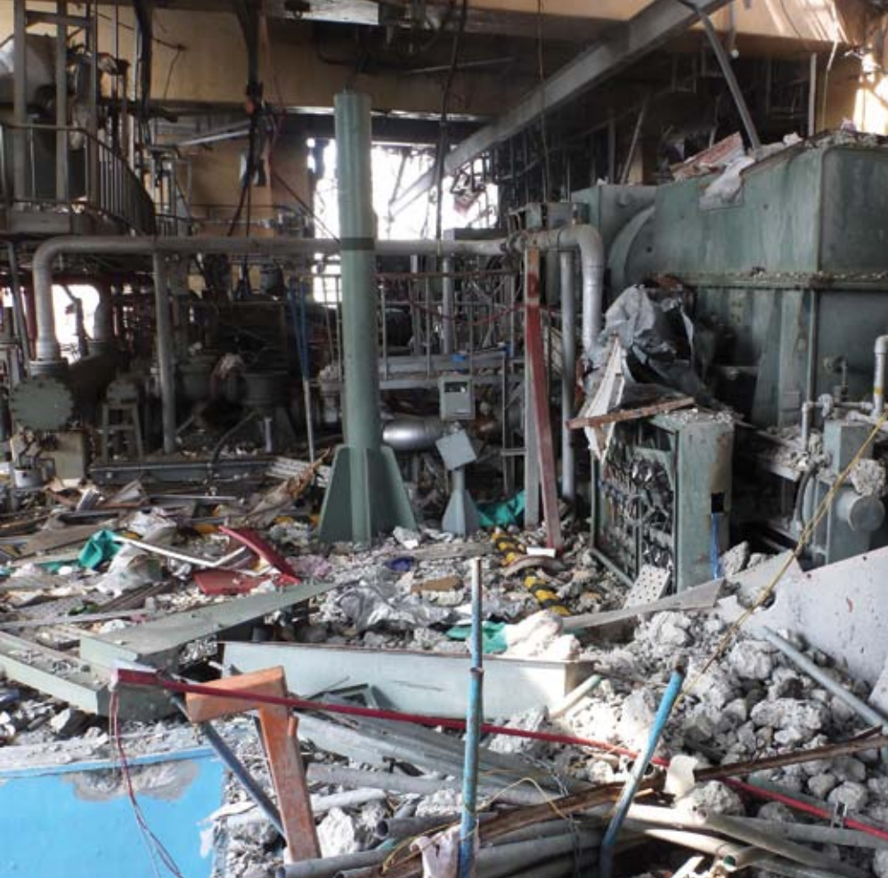
The Fukushima nuclear power plant's radiation recordings went off the scale in August 2011
